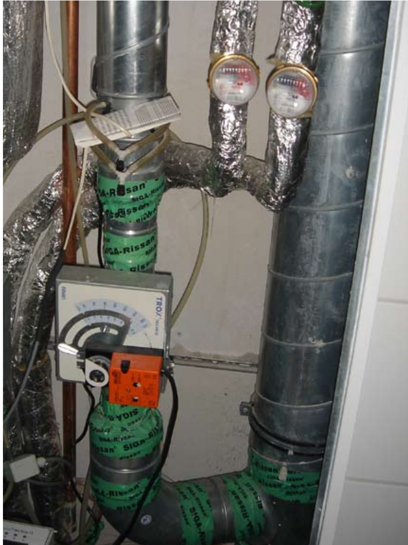
Technical installations, passive house in Hamburg, Telemannstraße
